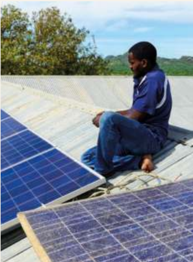
Installation of solar panels on the roofs of Loyoro village. Karamoja, Uganda, 7 April 2018.
